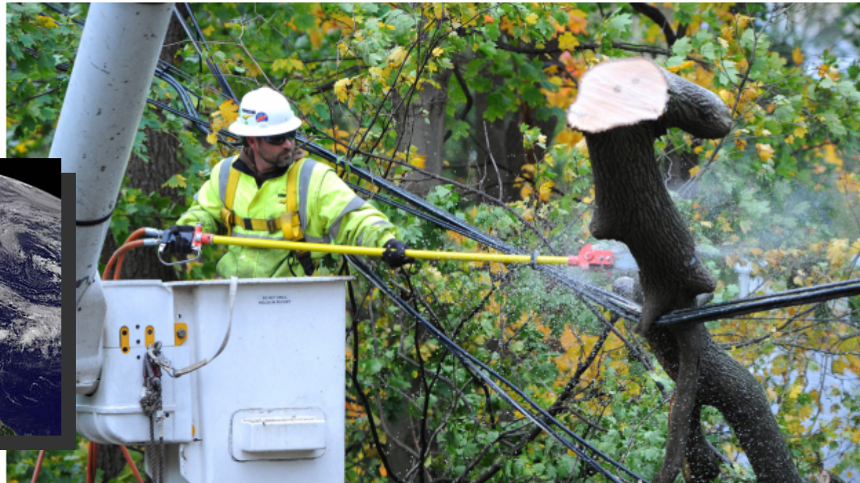
Matt Moran, a trimmer with Townsend Tree Service, cuts a fallen tree limb from a power line on 19th Avenue that fell as a result of the strong winds from Hurricane Sandy, Monday, Oct. 29, 2012, in Sea Cliff, N.Y. / AP PHOTO/KATHY KMONICEK
